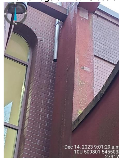
Photo 4: Cavities Adjacent to Previous Repairs
