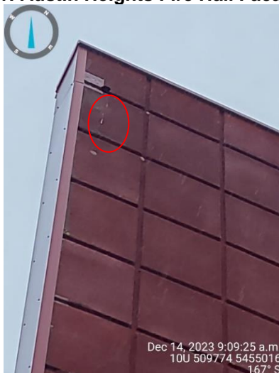
Photo 3: Whitewash Directly Below Cavity
