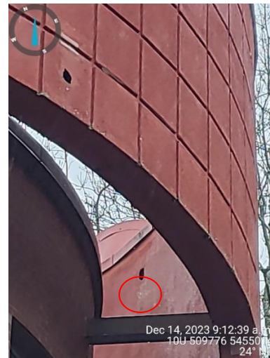
Photo 2: Bird Damage on Both Sides of Facade
