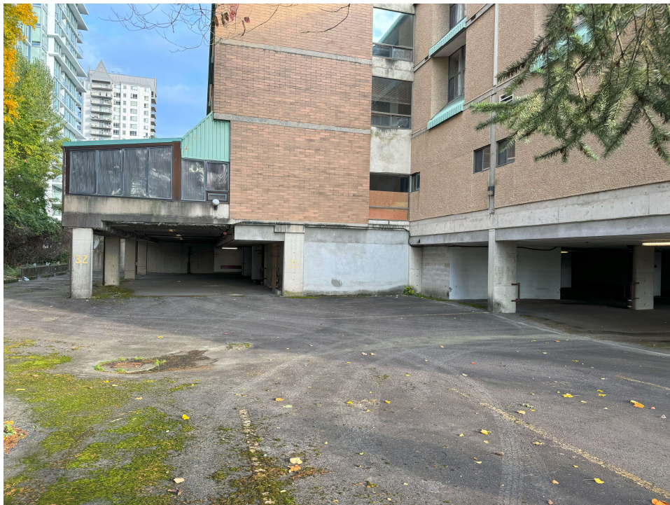
Photo 4 View north, showing walk out to ground level at the southern and western side of property.
