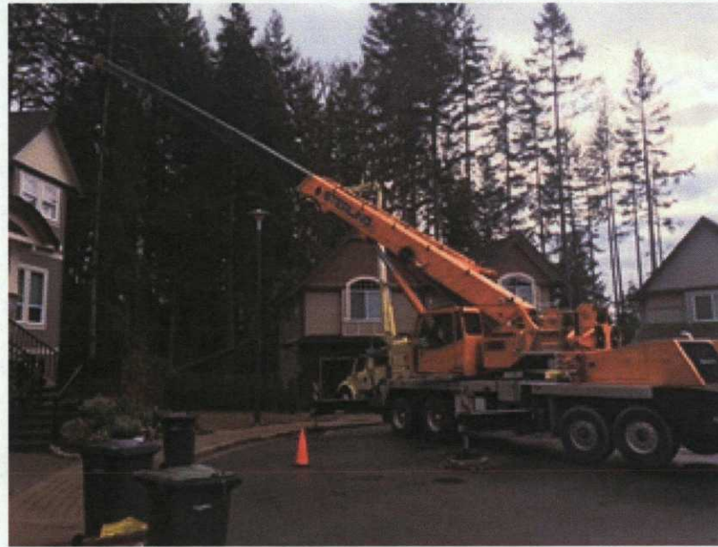
Crane required to remove a fallen tree from a home
