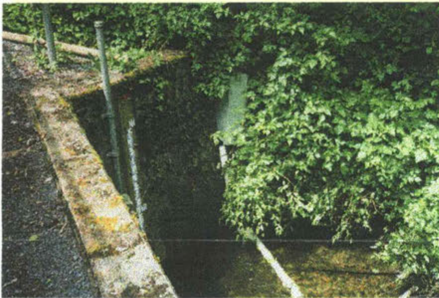
HYDROMETRIC KIOSK MOUNTED ON ABUTMENT WITH PVC SENSOR EXTENSION
